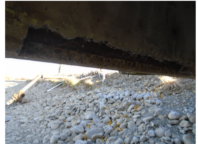
Eroding concrete girder
